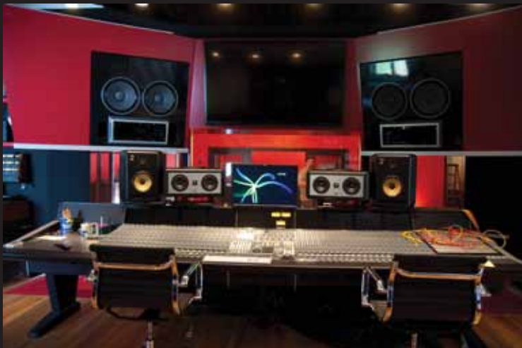
Kid Rock Studio A - Designed & Technical Install SSL Duality 48 Chan with Custom GBP G215K Monitors (Soffit Mounted)
