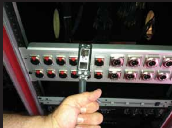
Custom Connector Panel Design & Fabrication
